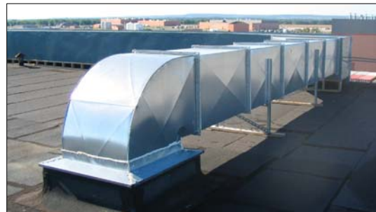
Above, the heat from the SolarWall panels is ducted across the roof to the building rooftop air intake and HVAC system.
